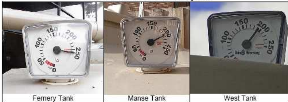
Tank Water Levels at 18 th February 2010
