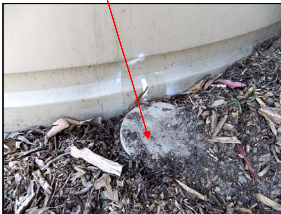
West side outlet to Fernery Pump
