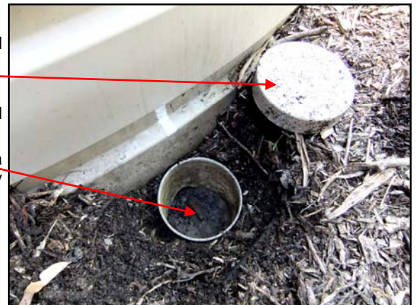
West side outlet to Fernery Pump
