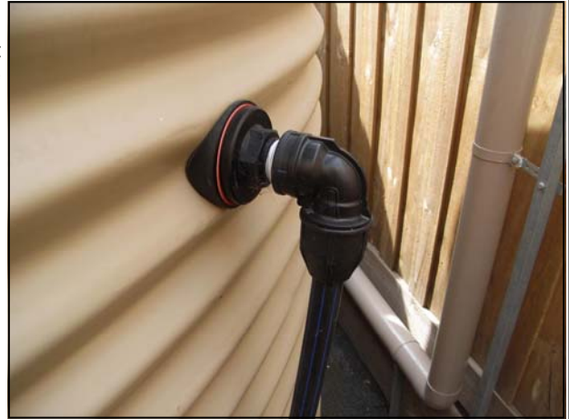
Fig 3.27 - Manse Tank float Valve
