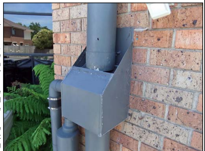
Fig 3.32 - Downpipe Filter, (final arrangement)
