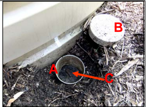
Fig 3.46 - Fernery Tanks isolation valves, Valve pit (A), cover removed (B) & valve at bottom (C)
