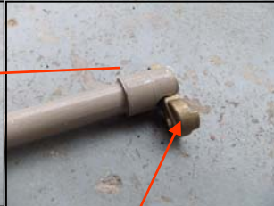
Fig 3.48 - Valve handle (removed from valve)
