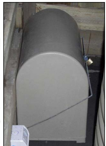
Fig 3.26 - Manse Pump Cover
