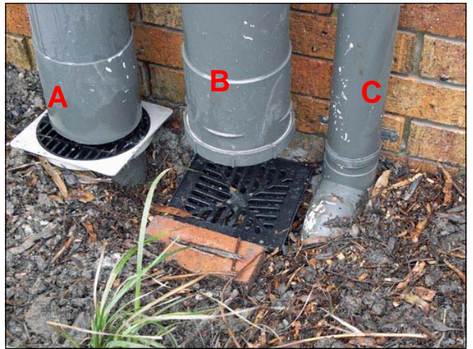
Fig 3.33 - First Flush Filter in place
