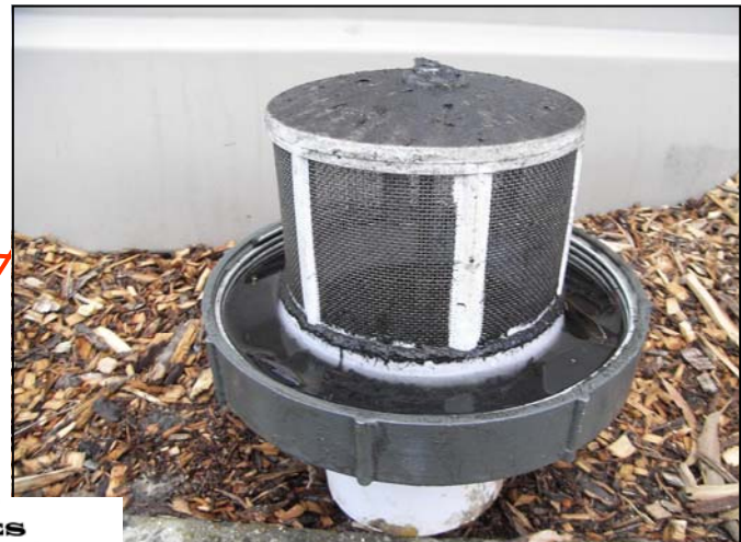
Fig 3.34 - Filter removed for cleaning
