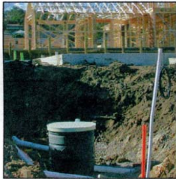
Installation of an Atlantis® Filtration Unit in the garden area of new home.
