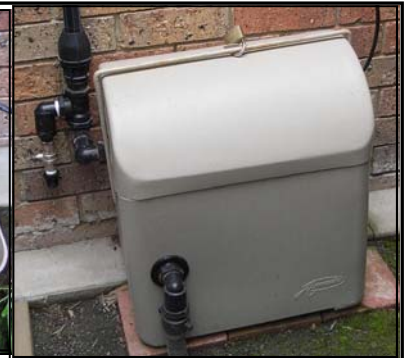
Fig 3.9 - West Pump, enclosure
