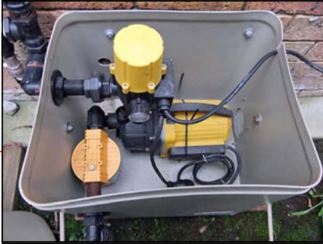
Fig 3.11 - Inlet Filter in enclosure
