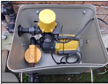
Fig 3.8 - West Pump, Lid removed
