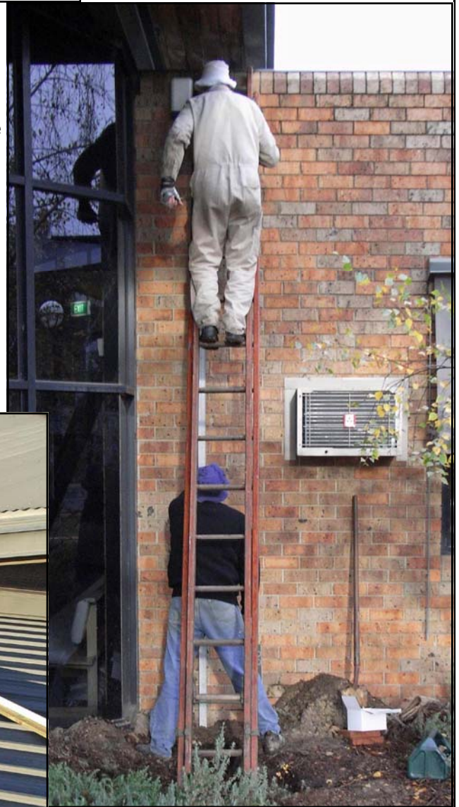
Fig 1.5 - Pipe route up Office wall
