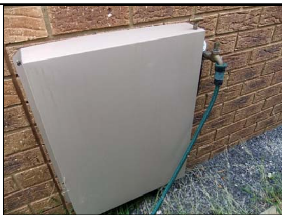
Fig 1.54 - Valve Train with adjacent Tank Water Tap
