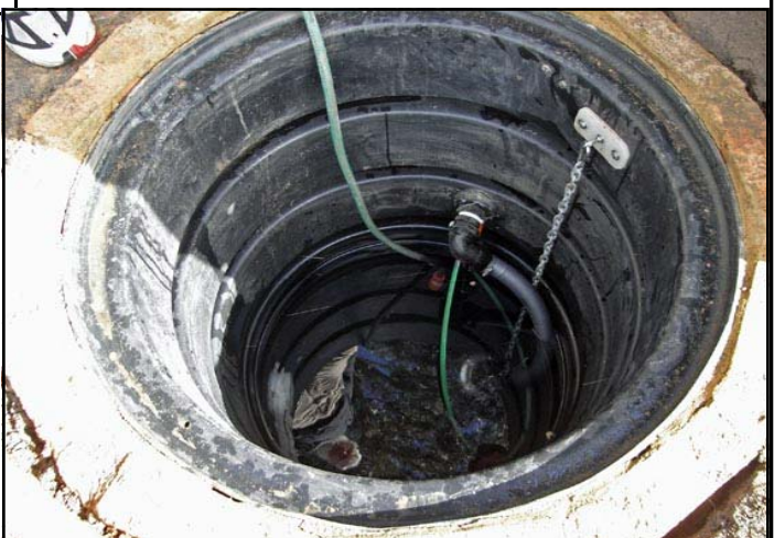
Fig 1.3 - Pump Pit with Pump at lower RHS
