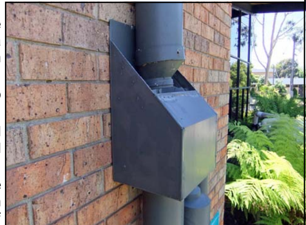
Fig 1.48 - Vestry Downpipe Filter
