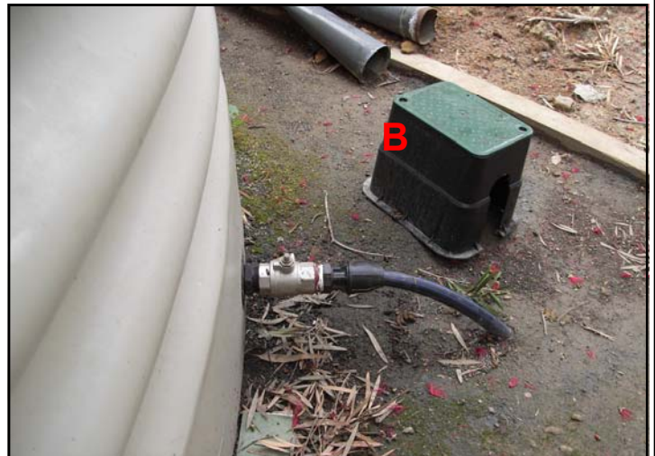
Fig 1.34 - Tank Isolating Valve (on West Tank) to
