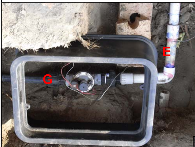
Fig 1.65 - Garden Watering Main Solenoid Pit C
