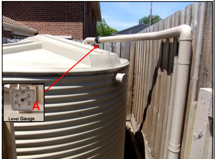
Fig 1.40 - Manse Tank, 8,000 litres
