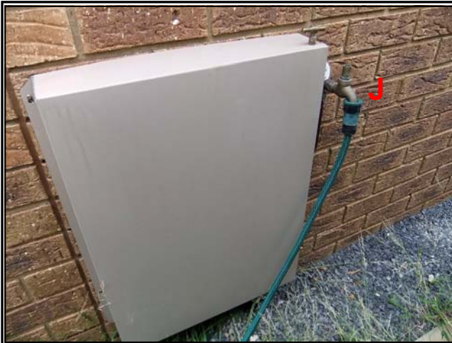
Fig 1.46 Valve Train with cover in position and adjacent "test" Tap
