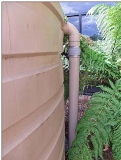
Fig 1.55 - Fernery Tank Overflow
