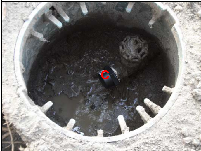
Fig 1.64 - Pit B Solenoid Valve removed
