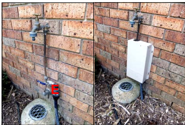
Fig 1.58 - Water Tap upstand & Mains Water to Fernery Pump, without & with valve cover
