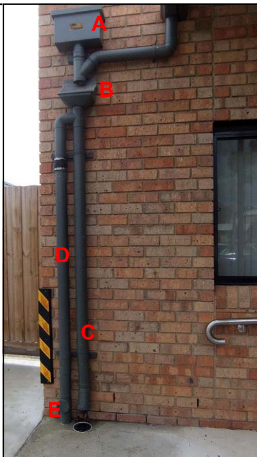
Fig 1.35 - Hall extension rainhead at south – east corner, downpipe & filter, 1st Flush, drain & grate, & Wet Leg
