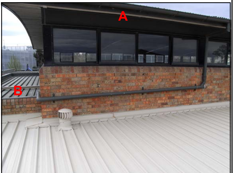
Fig 1.21 - Water from Hall and Store Roofs
