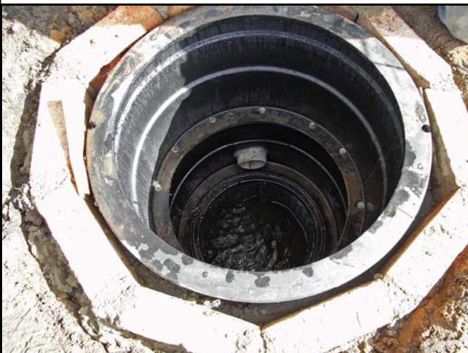
Fig 1.2 - Filter Pit with basket removed
