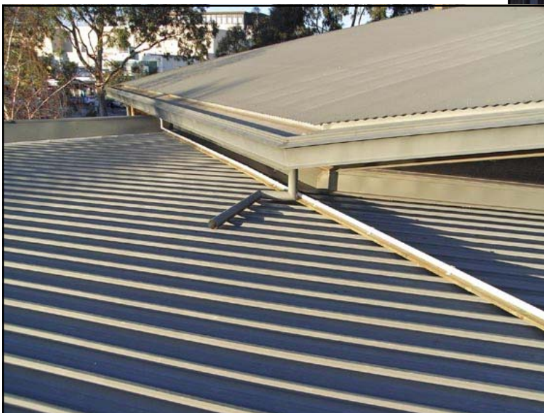
Fig 1.6 - Pipe route across Foyer roof
