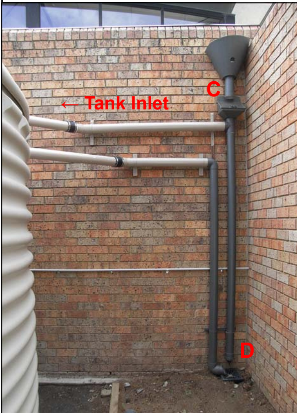
Fig 1.22 - Downpipe Tank inlet, filters & Tank overflow West Tank
