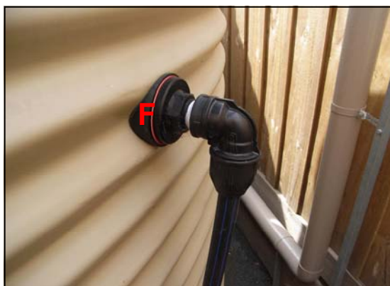
Fig 1.38 - Gravity line connection to Ball valve inside Manse Tank
