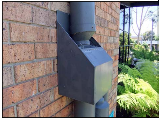
Fig 1.48 - Vestry Downpipe Filter
