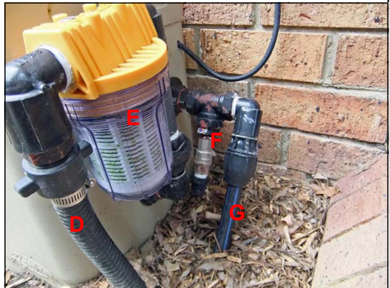
Fig 1.60 - Fernery Pump with cover removed
