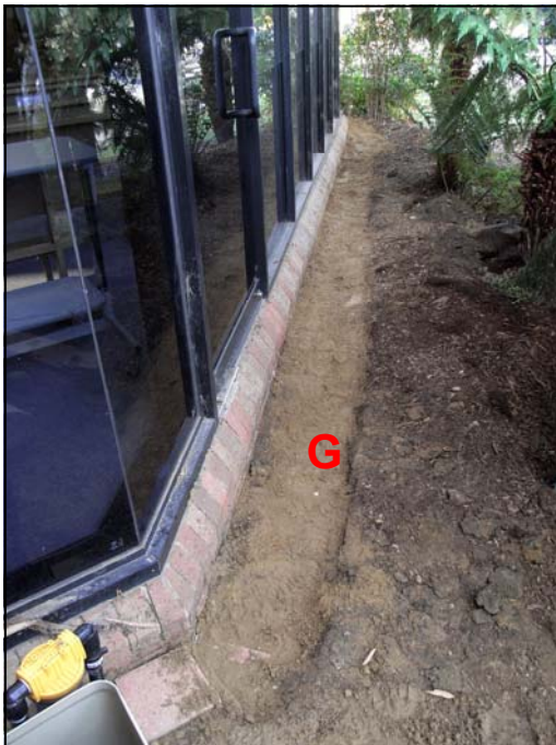
Fig 1.61 - Pipe route from Pump
