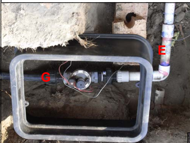
Fig 1.65 - Garden Watering Main Solenoid Pit C
