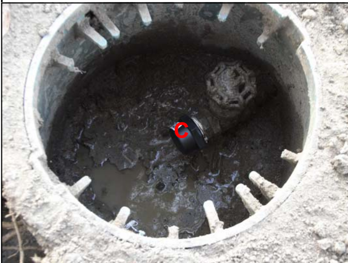
Fig 1.64 - Pit B Solenoid Valve removed
