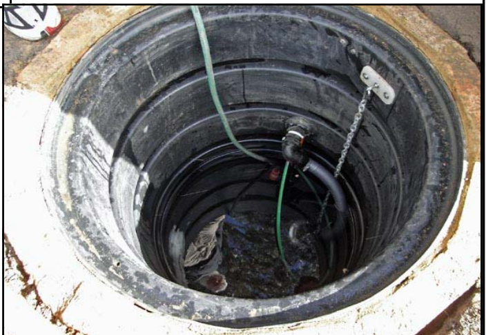
Fig 1.3 - Pump Pit with Pump at lower RHS
