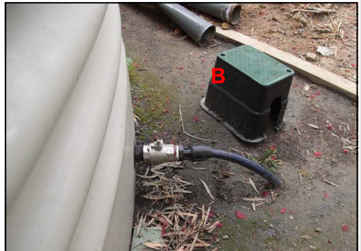
Fig 1.34 - Tank Isolating Valve (on West Tank) to
