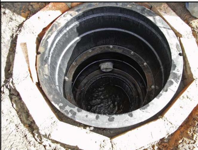
Fig 1.2 - Filter Pit with basket removed
