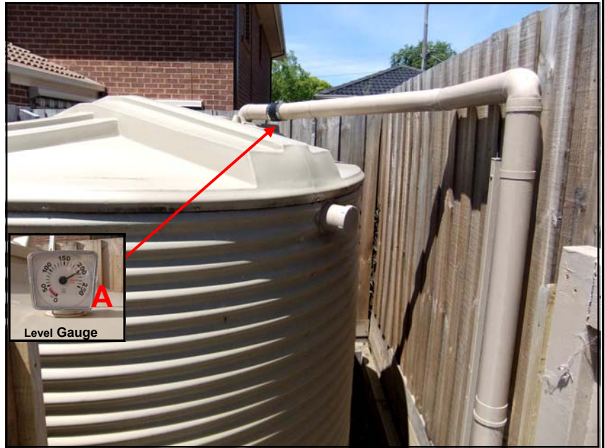
Fig 1.40 - Manse Tank, 8,000 litres
