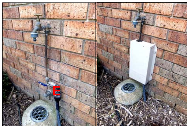
Fig 1.58 - Water Tap upstand & Mains Water to Fernery Pump, without & with valve cover
