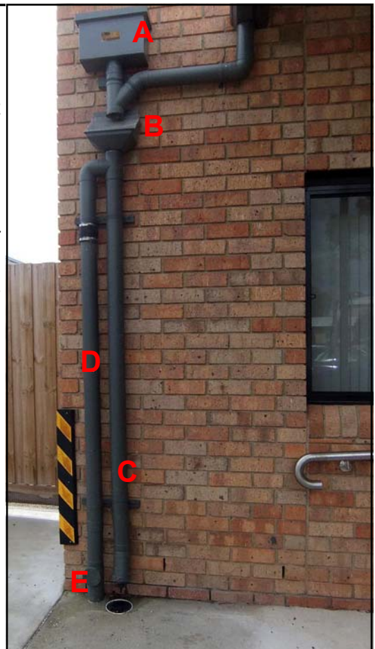
Fig 1.35 - Hall extension rainhead at south – east corner, downpipe & filter, 1 st Flush, drain & grate, & Wet Leg
