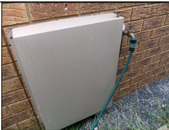
Fig 1.54 - Valve Train with adjacent Tank Water Tap
