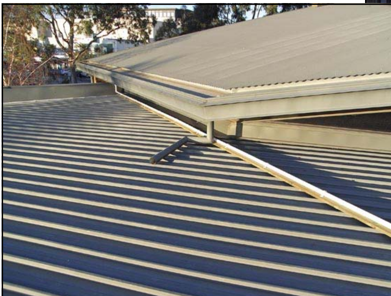
Fig 1.6 - Pipe route across Foyer roof
