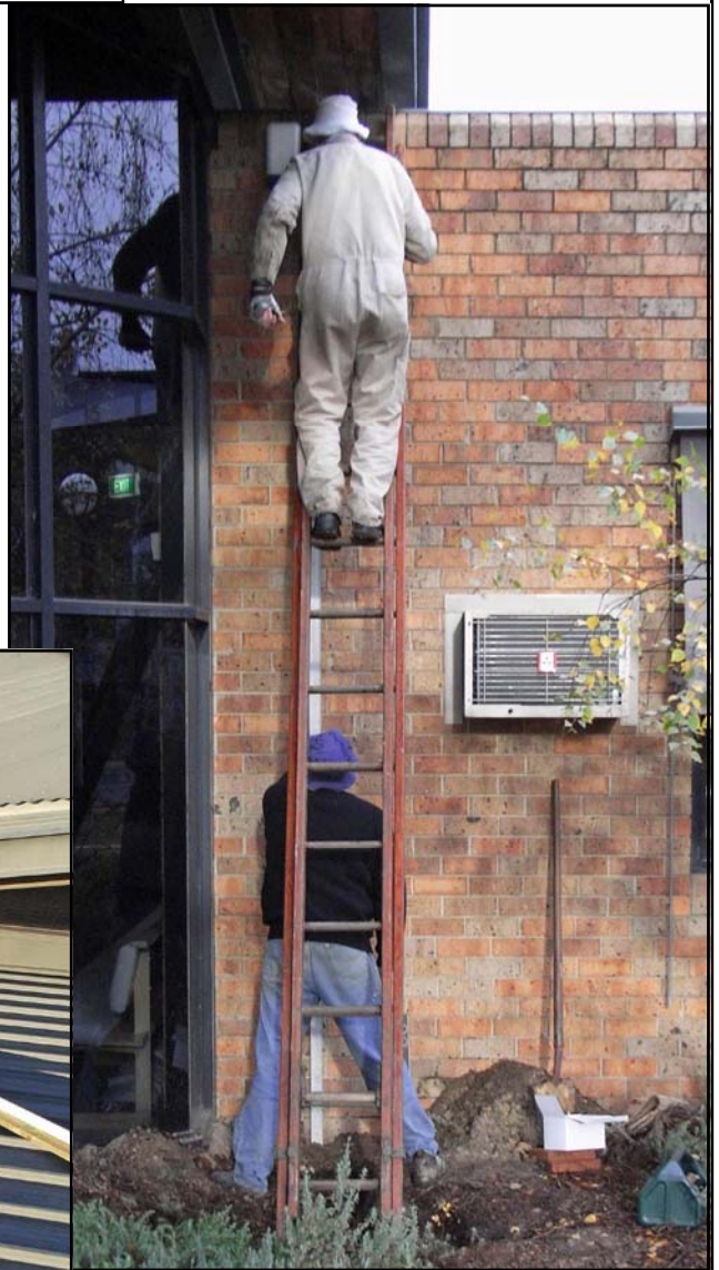
Fig 1.5 - Pipe route up Office wall
