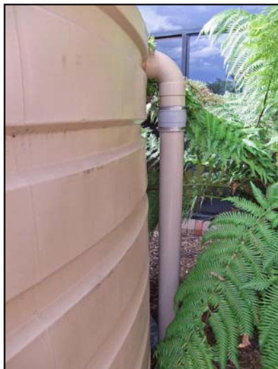
Fig 1.55 - Fernery Tank Overflow
