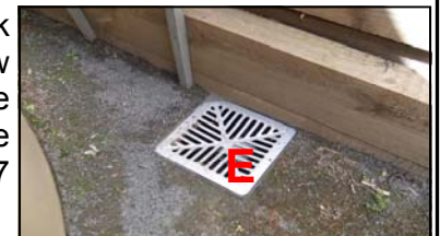
Fig 1.39 - Storm Water Pit, Manse Tank area
