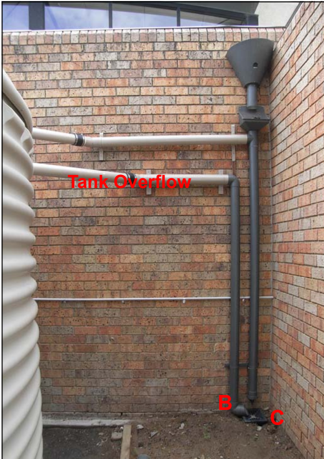
Fig 1.28 - West Tank overflow & stormwater drain
