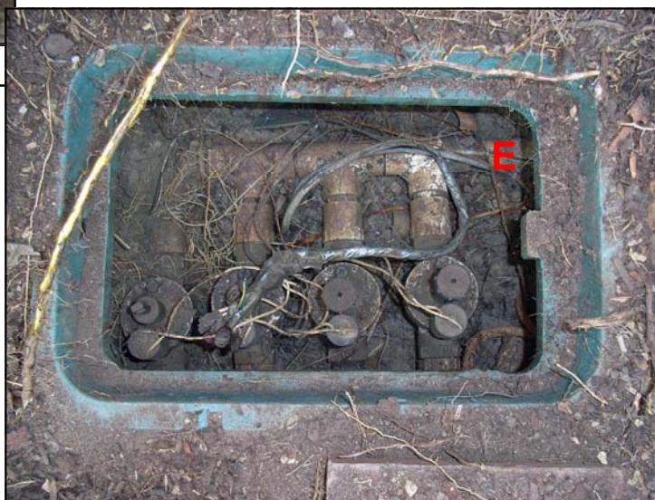
Fig 1.66 - Garden Watering East , 4 Solenoid Valve Pit
